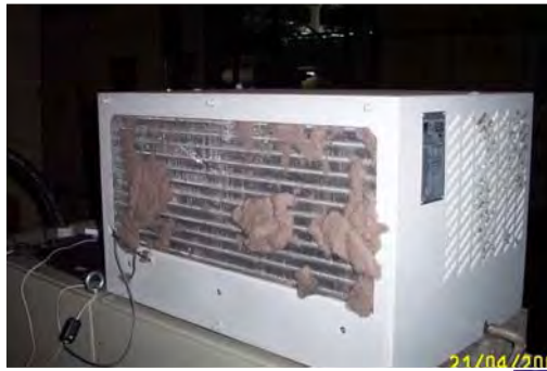
Heat exchanger without coating in textile industry
